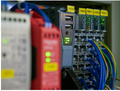
Control SPS moderno
